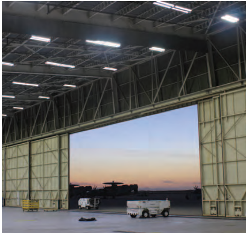
The new lighting system will include daylight sensors that dim in the presence of adequate natural light.
