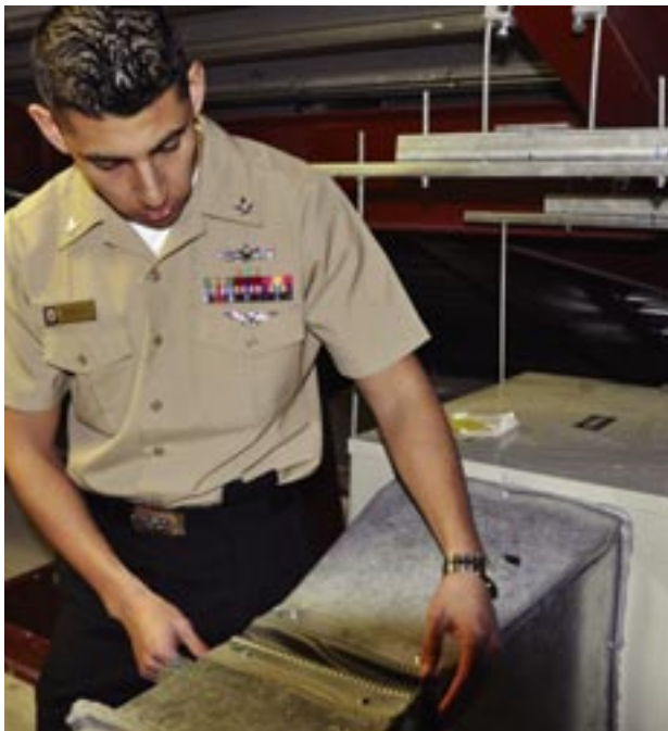
Air duct inspection at Naval Station Rota in Spain. Many energy efficiency improvements are low cost and generate ongoing revenue from the resulting savings.
