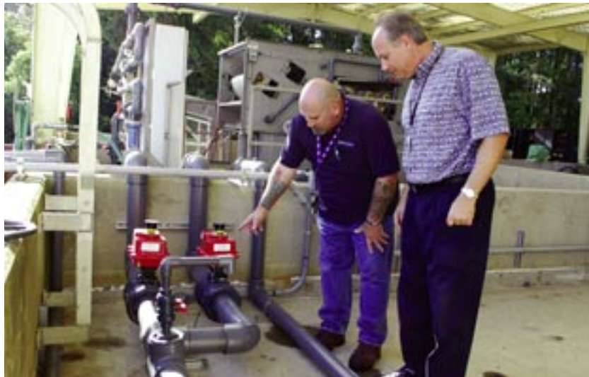
Casey Cochran, utilities supervisor for Richard Brady and Associates, left, points out some of the unique functions of the solenoid valve for the Clean B Solution to Jay Caddy, commodity manager for NAS Jacksonville Public Works Utilities and Energy Management. The valves filter the water for after it is disinfected either into the Chemical Sludge Treatment System or back to the wastewater treatment plant to be retreated.
