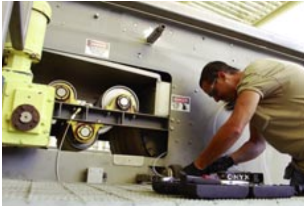
Kevin Savela, general maintenance worker with Richard Brady and Associates, works on the air system of the belt filter press at the Wastewater Treatment Plant.
