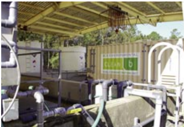
The Chemical Sludge Treatment System, tanks and components treat an average of 40 gallons per minute of waste sludge from the NAS Jacksonville Wastewater Treatment Plant.
