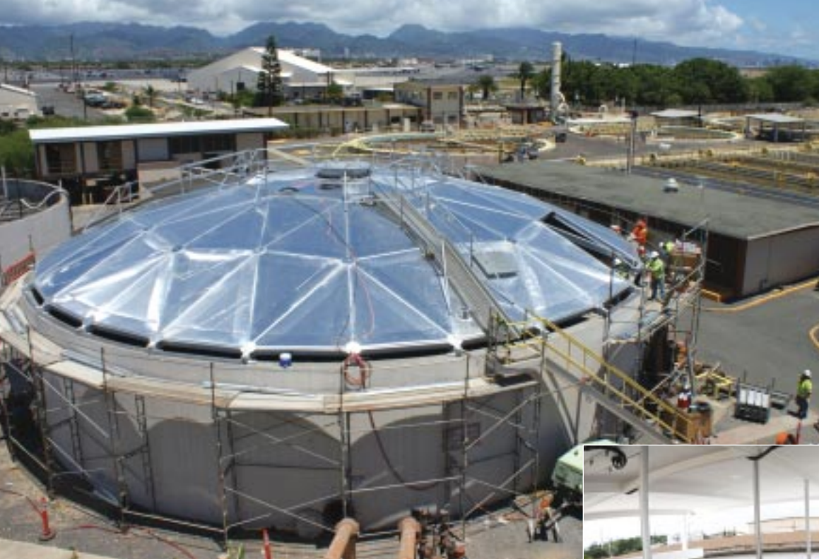
Naval Facilities Engineering Command Hawaii is upgrading the wastewater treatment plant at Joint Base Pearl Harbor-Hickam by removing the floating steel roofs and replacing them with fixed aluminum dome covers. The new covers will help capture methane gas for future energy projects and use it as an alternative fuel source. Denise Emsley
