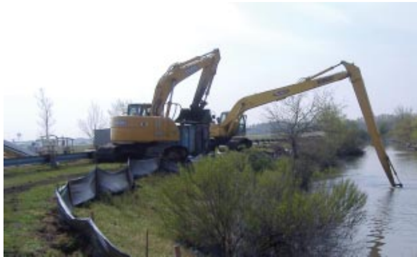
Excavation activities in the section of Bousch Creek adjacent to the NSN flight line. Excavation was completed from the top of the bank with a long-reach excavator to avoid impacting established vegetation along the banks. The depth of excavation was measured using a man lift located on the top of bank to avoid having workers in the water.
