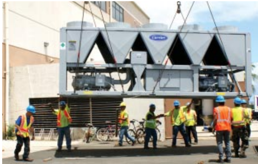
The installation of new energy efficient air conditioners at NAVSTA Pearl's Building 1770 is saving more than $92,000 annually.
