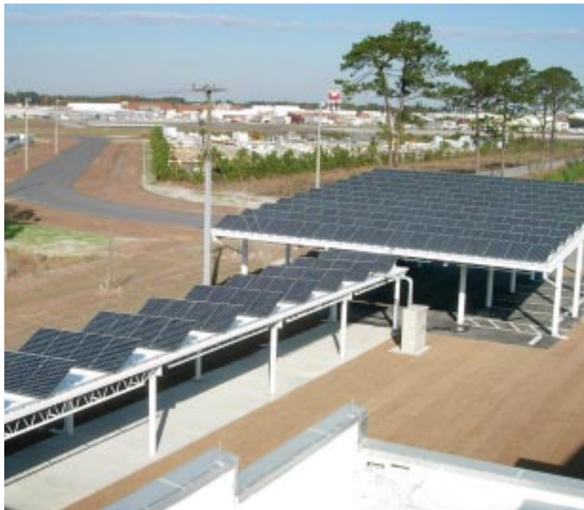
The photovoltaic panels added to the new Engineering Product Support Facility at FRC East helped to move the project from LEED Silver to LEED Gold certification. These panels provide a clean, renewable energy source for 23 percent of the facility's energy use.
