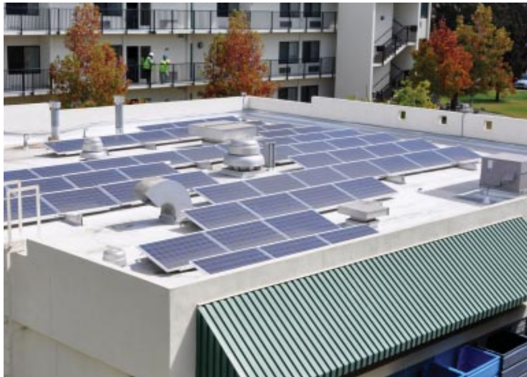
In 2010, NBSD funded and executed numerous photovoltaic projects to reduce energy use. These projects are achieving a positive return on investment through reduced energy consumption.
