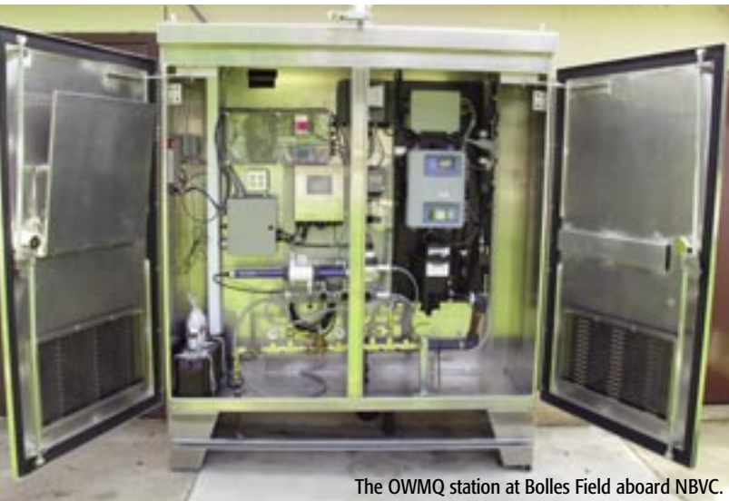
The OWMQ station at the Pleasant Valley Gate—where the water main enters NBVC.
